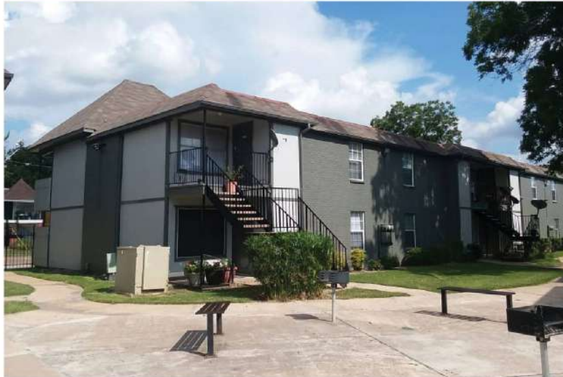
Demo & Rebuild | Apt Bldg | Houston, TX General Contractor | 8 units Bldg Jan 2020 - May 2020
